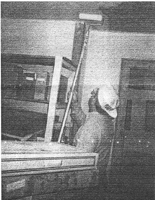
Andy Valerio paints the ceiling of the newly restored second floor storage room in the John Hunt House.
