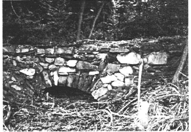
The work crews that cleared out the area behind the Hunt House uncovered the foundation to the bridge that once led to the Hunts Mills Amusement Park.
